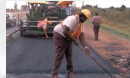
Road crews on the 4-Lane expansion on Highway 61 North from Cleveland to Clarksdale
