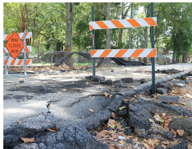
Roads across the South Delta are crumbling and caving in due to prolonged backwater flooding; Shell Beach Drive in Eagle Lake.
