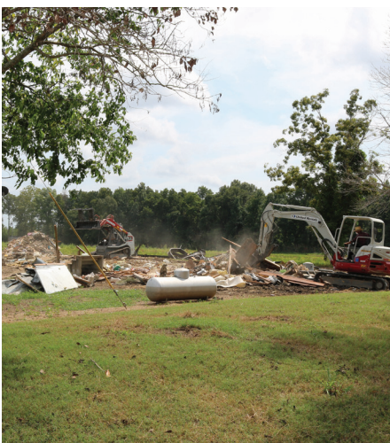
The Mennonite Disaster Recovery team demolished a family home on Diggs Road near Fidler destroyed by backwater flooding.
